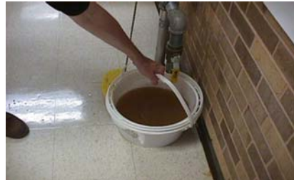
Unfortunately for Brent, the eyewash that he used had not been flushed for some time. This is the water that came from the eyewash after it was flushed.
